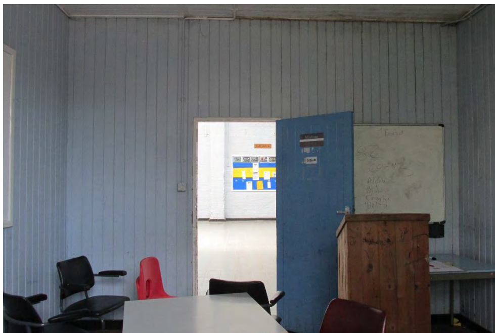
Figure 25: The blue painted panelled walls of the classroom, showing some mould to the top right corner, looking east
