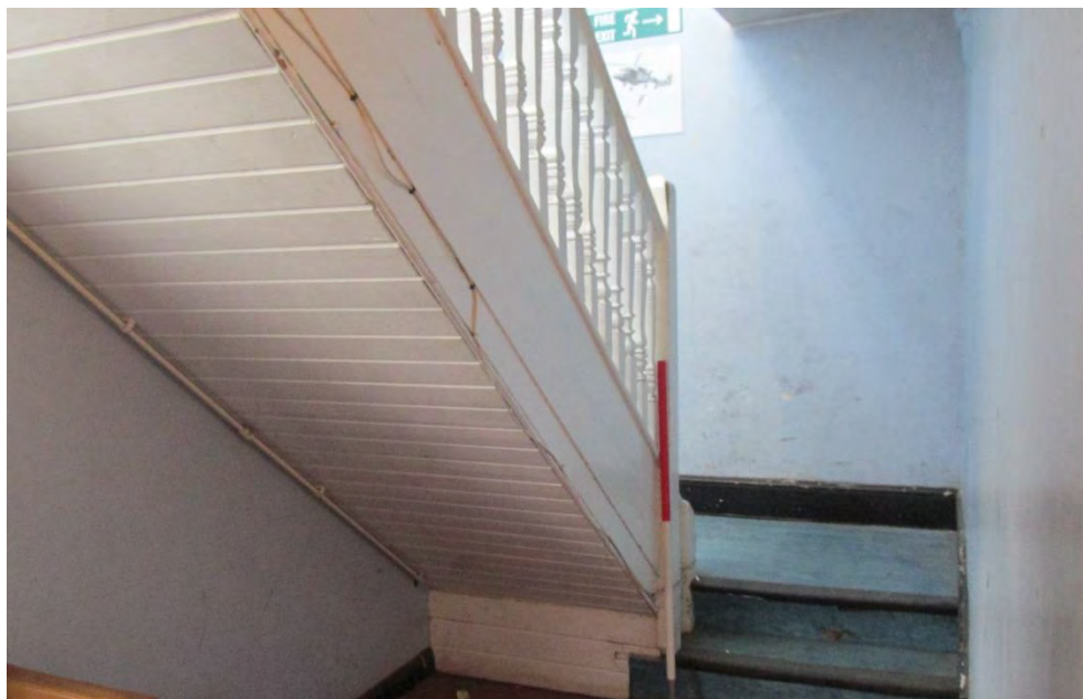
Figure 38: North west stairs, with small earlier pipe seen in top right, looking west
