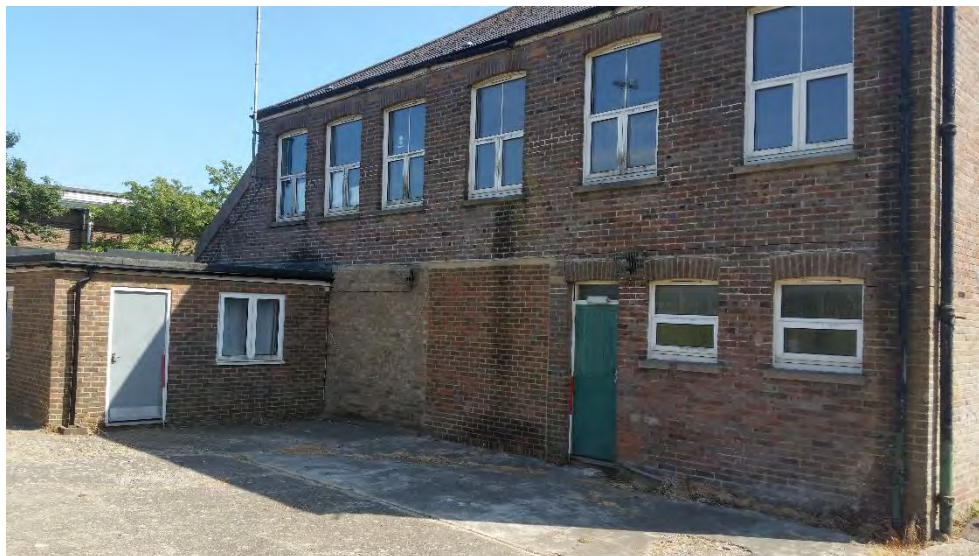
Figure 10: Rear elevation, showing the original window openings and new PVC windows, modern extension, as well as the filled in entrances to the cart stores east of the ground floor doorway, looking east
