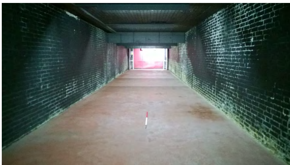
Figure 32: Looking down the rifle range, toward target, looking north. Some water damage to east wall seen here
