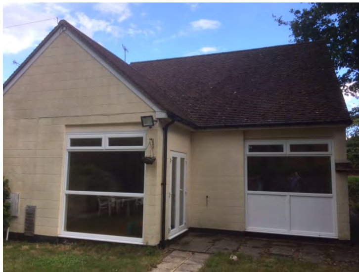
St. Francis Fields, Northiam - renovation of two bungalows in preparation for letting using CIL allocated in 2019/20
