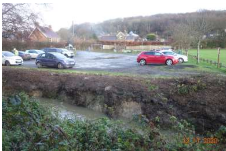
Powdermill Stream showing erosion by the car park (taken from the FP).
