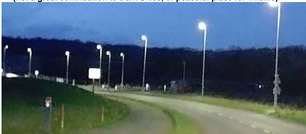
Carriageway lights between roundabouts
